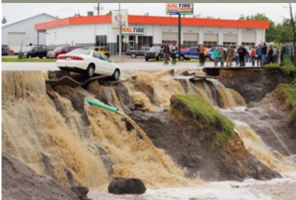
Exhibit 19: 2016 flooding in Dawson Creek
